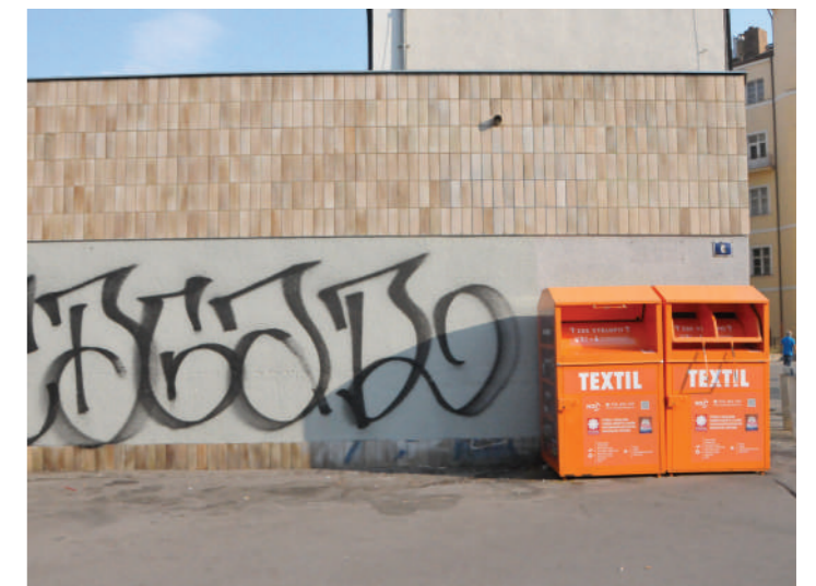
Graffiti on the facade, looking towards Ke Stvanici street
