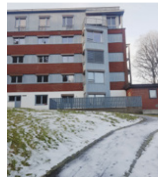
Photo shows facade and cladding at at the east side next to the garden. There has been additional attachments made to the existing building.
