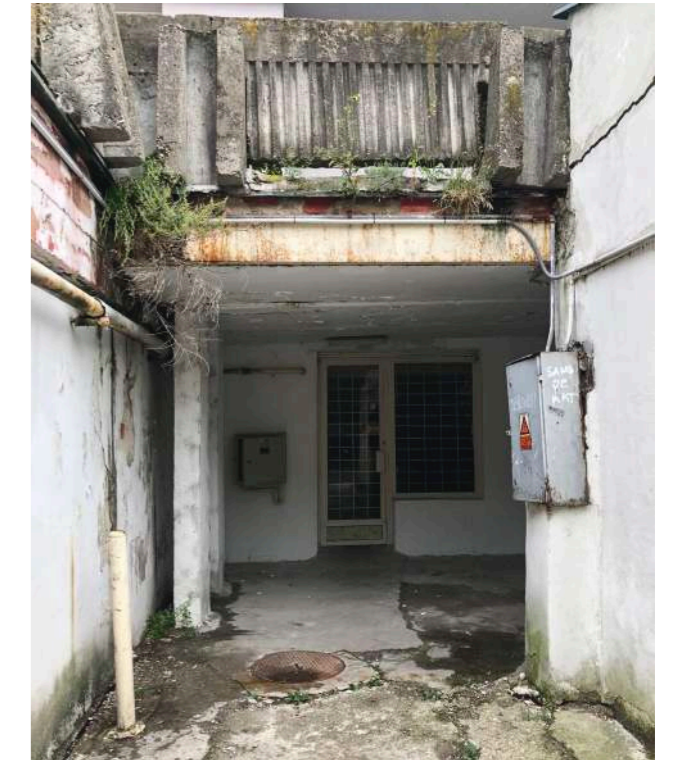
Lack of building maintenance.
