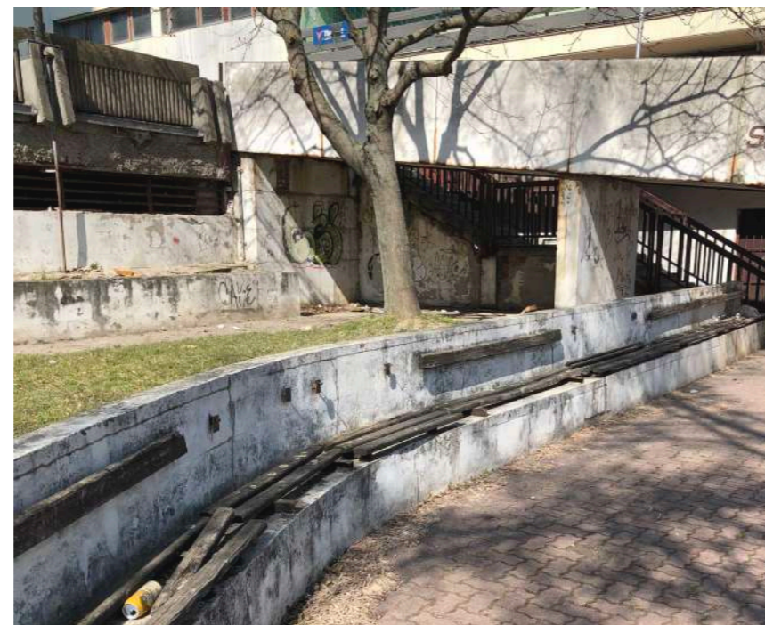
Unused public space lacking maintenance.
